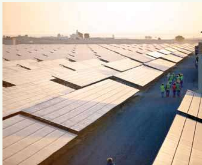
Figure 21: O&M Workers at a Large-scale Solar PV Power Plant
